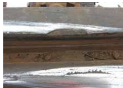
Typical wear damage
