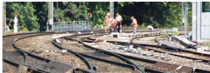
Checking switches on a track system
